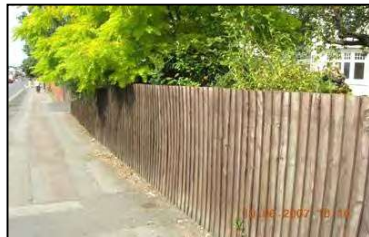
Figure 15 Poor wooden fencing on Hale's Road
