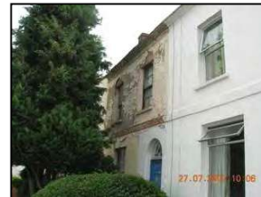
Figure 49 Façade of building in Fairview Street in need of maintenance
