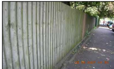
Figure 21 Poor fencing evident on College Road
