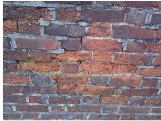
Figure 7. Bad example of pointing with cement mortar. Wide cement pointing prevents moisture escaping through joints, causing bricks to crack and lime mortar to erode.
