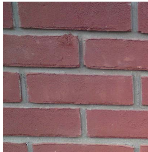
Figure 6. Good example of new facing brickwork. Showing slightly recessed pointing with the faces of the brick kept clean of mortar.
