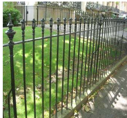
Good example of replacement railings, with tulip bud and urn finials set in Forest of Dean sandstone plinth. Railings are located outside Summerfield House, Bayshill Road.
