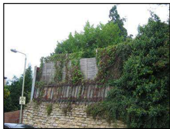
Figure 54 Poor boundary treatment on junction of Cudnall Street with Overbury Street
