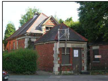
Figure 37 Derelict Charlton Kings Village Hall
