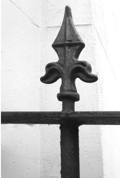
Fig.19 Mismatched railing finial, Suffolk Square
