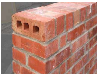
Fig.23 Use of header course in place of coping stones, Marle Hill Parade
