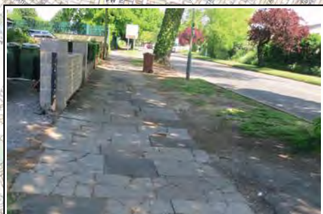
1. Cracked and uneven sections of paving along sections of Hewlett Road and Priors Road.
