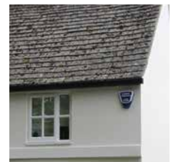
Fig.6.3 Introduction of alarm boxes
