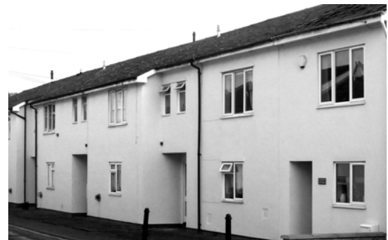
Fig.25 The effect on a terrace of an unbroken expanse of roof, Park Street
