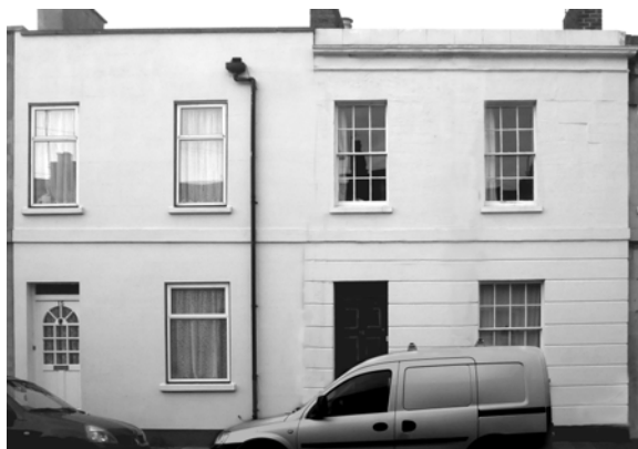
Fig.14 The effect on appearance due to the loss of original entablature, windows and door, St Paul's Street North
