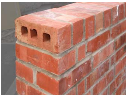
Fig.23 Use of header course in place of coping stones, Marle Hill Parade
