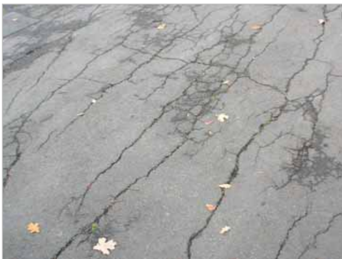
2008 Cracked surface on Pump Room Drive
